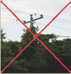
OVERGROWN VINES AROUND ELECTRICAL EQUIPMENT
